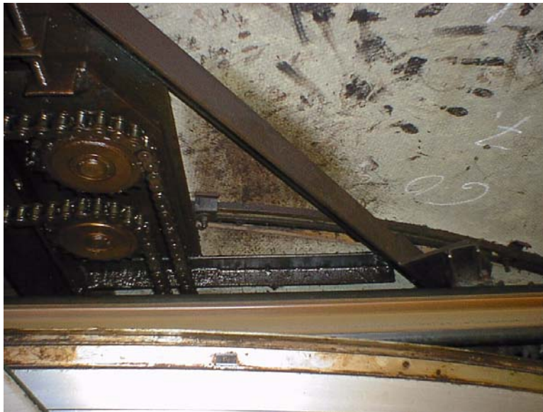
Side Panel on Escalator
