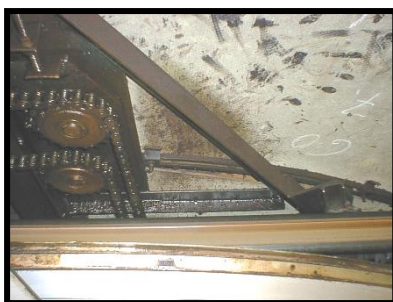
Asbestos panelling cladding escalator handrail drive adjuster
