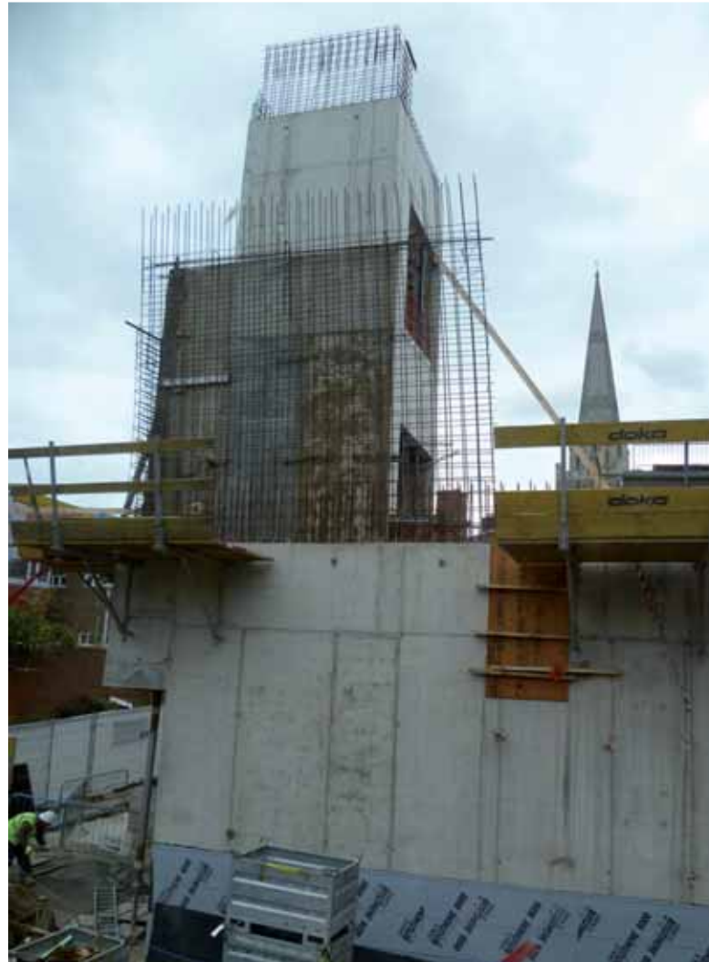
Soaring upwards: the liftshaft at The Novium and the ancient spire of Chichester Cathedral
